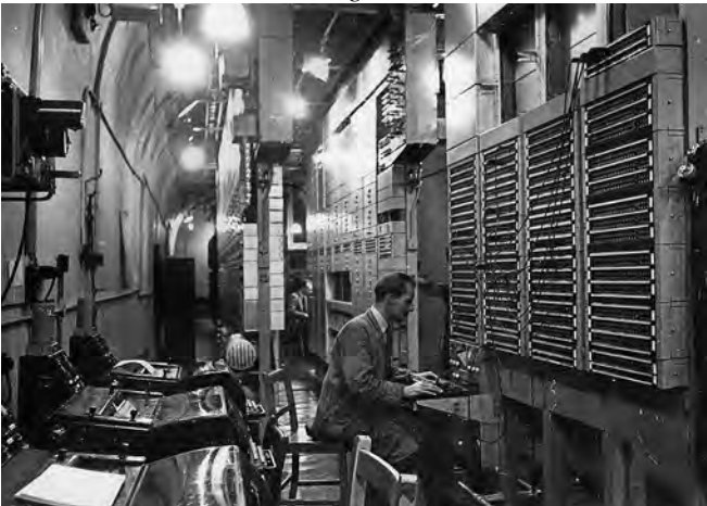
GPO telegraph equipment
